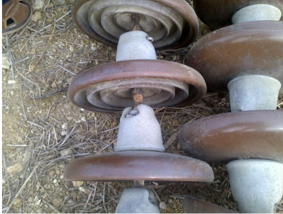
Figure 3. Sample of insulators deteriorated due to contamination
