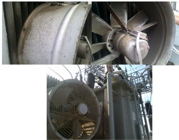
Figure 2. Deposition of the quarry dust in the fans of the substation
