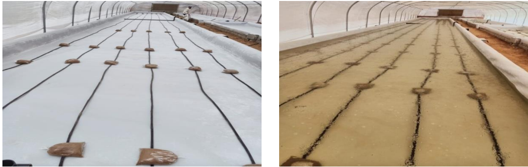
(a) Installation and preparation of the ventilation network for planting ponds (b) Testing the ventilation net before planting with porous polyurethane hoses
