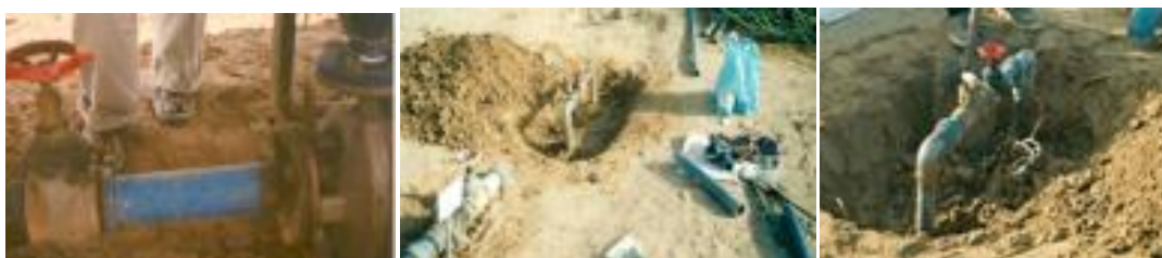
Figure 2. Irrigation systems networks maintenance.
