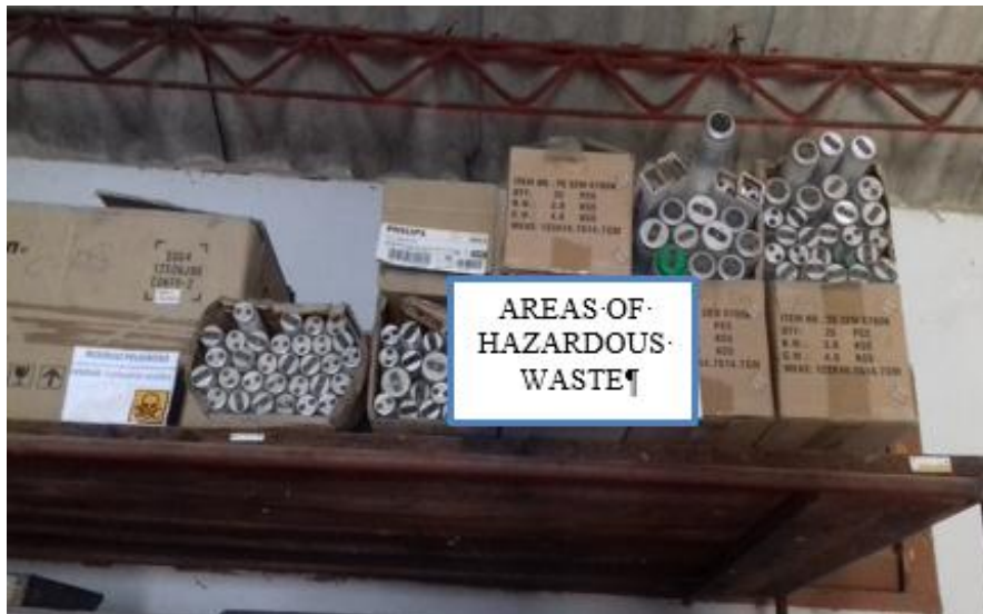
Figure 3. Area destined for the storage of the luminaires (UIC Santiago de Cuba)
