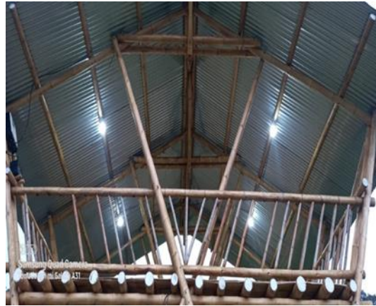
Figure 5. Recessed luminaires inside the reed
