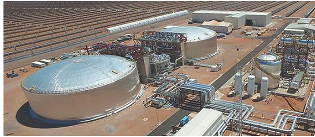
Figure 4. Storage tank Source: (Boese Franco, 2022)
