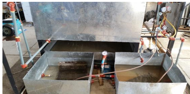
Figure 3. Chiller operating units
