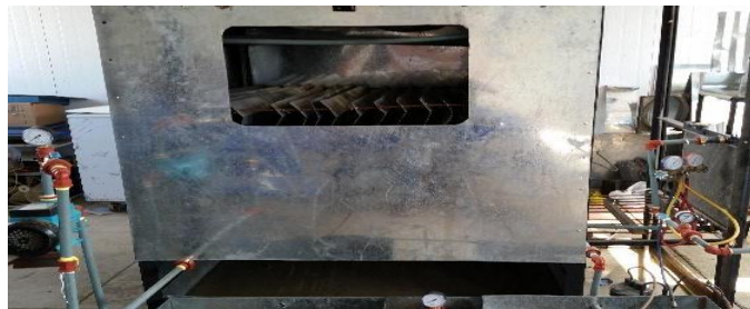
Figure 2. Chiller operating units
