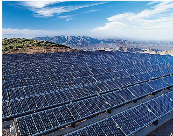
Figure 5. Solar park installed in Gonzanamá (2 MW)
