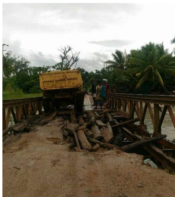
Figure 6. Ndalir Bridge damaged by high tide (personal documentation)
