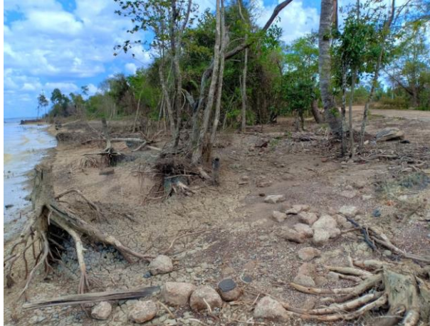
Figure 3. The old Ndalir village area that was damaged by abrasion (personal documentation)
